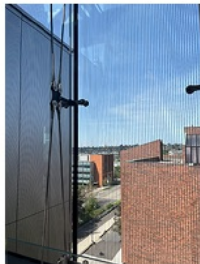
An example of bird-safe glass installed in the Life Sciences Building on the UW campus. Photo by Judy Bowes.
