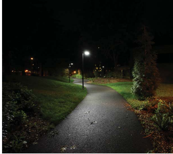
Figure 23. LED campus standard fixture along path adjacent to the Intellectual House.
